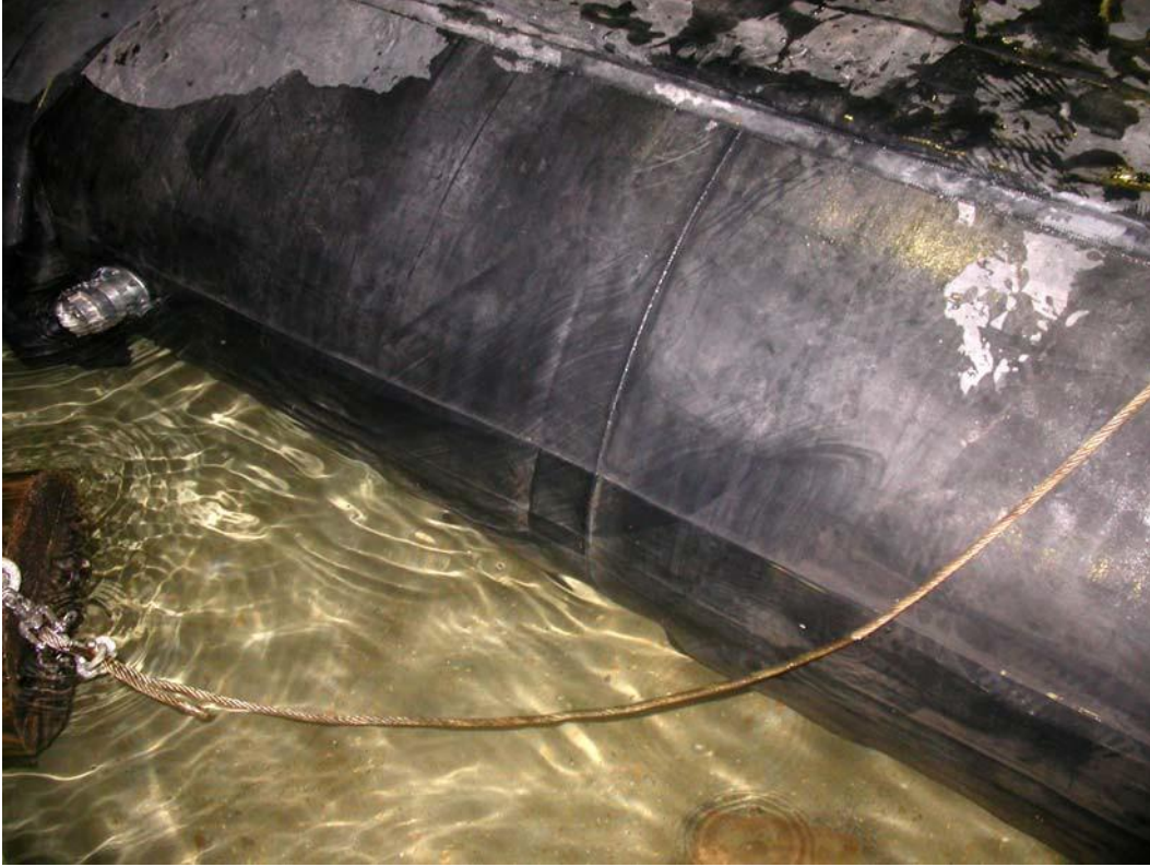
Figure 9. Twelve in log and location of impact on Unit B-2
